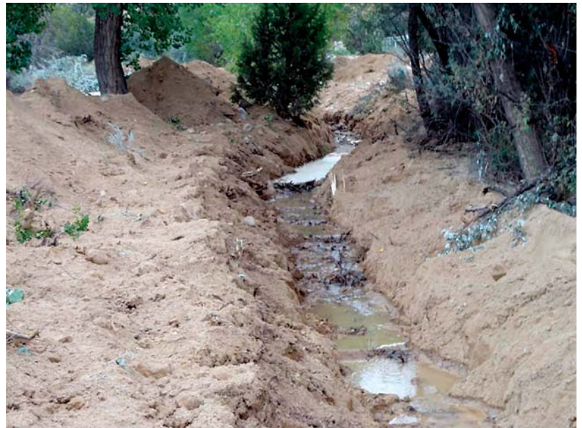
The first water in the ditch after repairs from the flooding in San Juan County on August 26, 2015. Photo by Earnest Smith, President of the Lower Animas Ditch Association.
