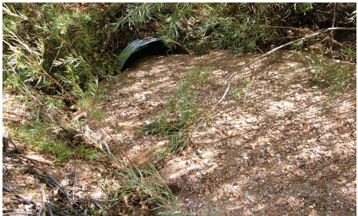
Acequia Potrero culvert after severe flooding in 2013.
