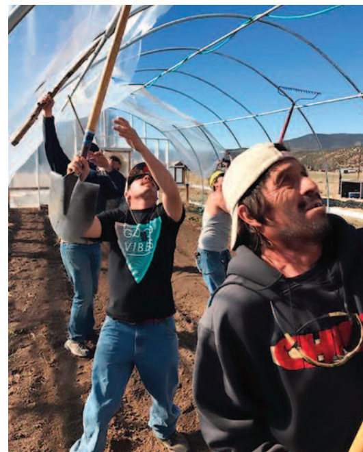
Los Sembradores Farmer Trainees building a high tunnel. Photo by Serafina Lomabrdi, NMAA Staff.
