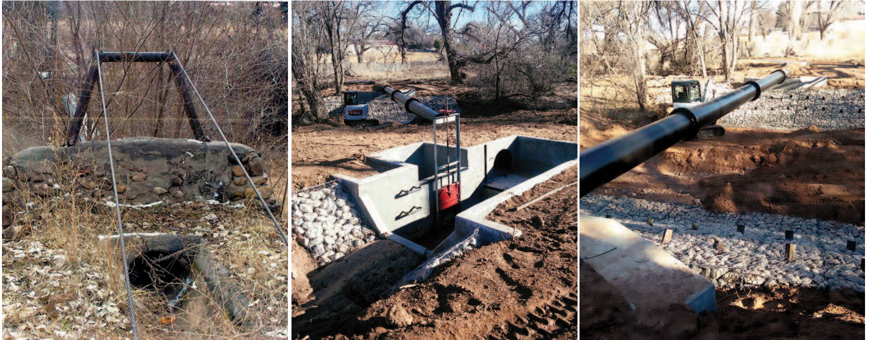
(l to r). The old infrastructure on Acequia de la Jolla, built in 1947. Acequia de la Jolla replaces an old flume with a self supporting steel flume in 2016. The Regional Conservation Partnership Program of USDA funded this infrastructure project; this vital funding would no longer be available under the proposed budget cuts. Photos by Edward Romero.
