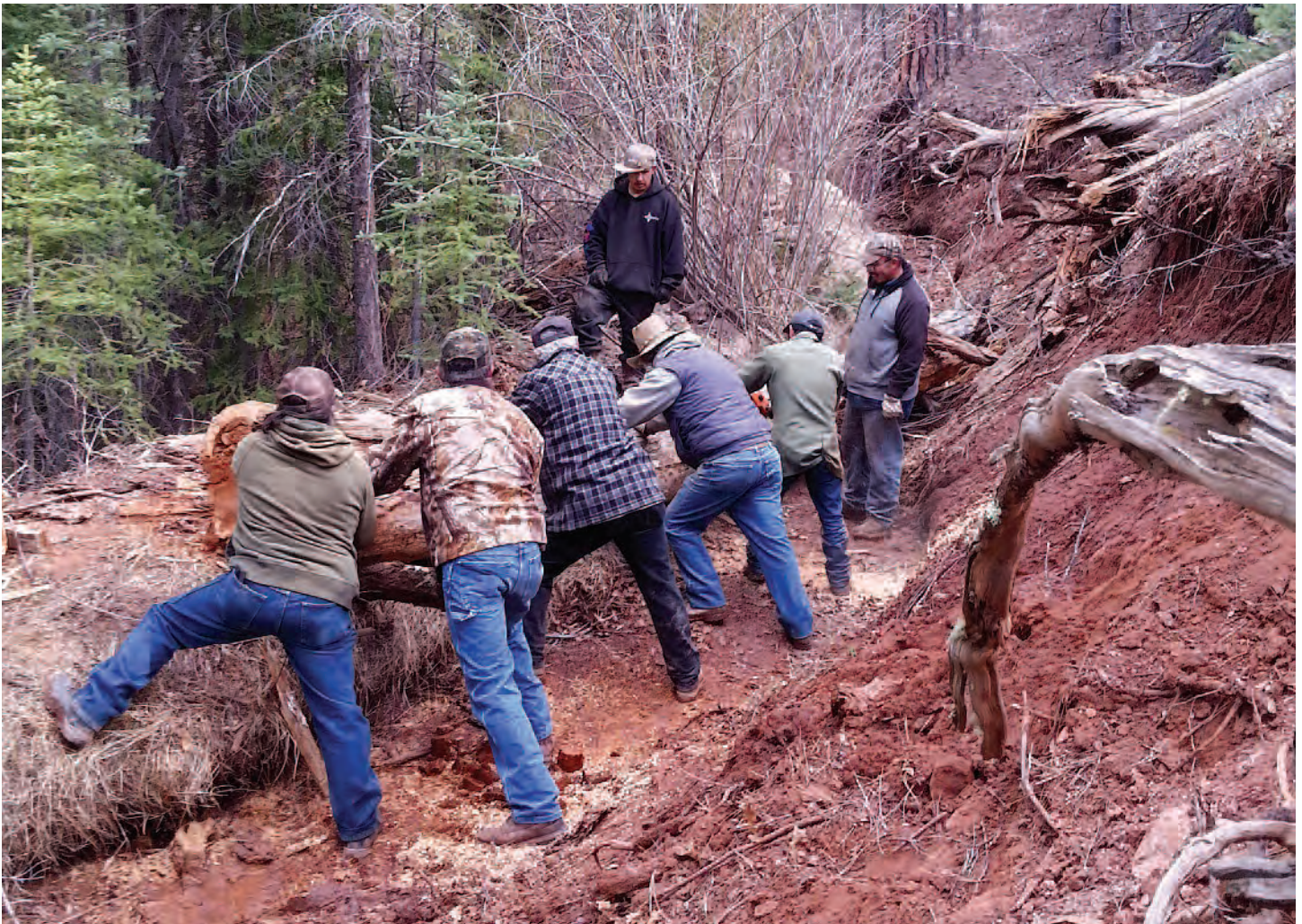
Good acequia parcientes and neighbors working together to clear the logs that fell into the Cecilia Ditch in Gallina, NM. Photo taken by Victoria Suzao-Chanza.
