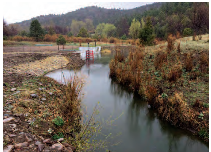
Acequia del Alto Al' Norte completed dam project. Photo by Paula Garcia.
